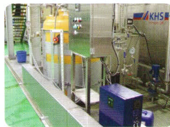
HOCL0.36t Line washing unit (Beverage factory)
